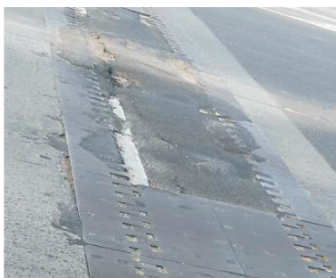
(b) 伸缩缝破损严重 (b) Seriously damaged expansion joints
