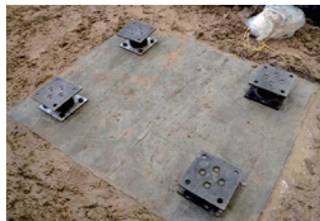
(a) 隔震支座的平面布置 (a) Plane layout of the isolation bearings
