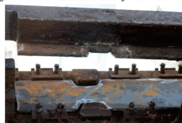
(b) 小车轨道垫板更换现场 (b) Site of trolley track pad replacement
