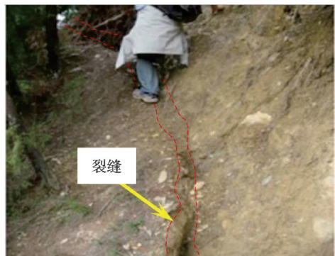
(b) 青川县红光乡三元坝边坡裂缝 (b) The crack of Sanyuanba slope in Hongguang town Qingchuan county
